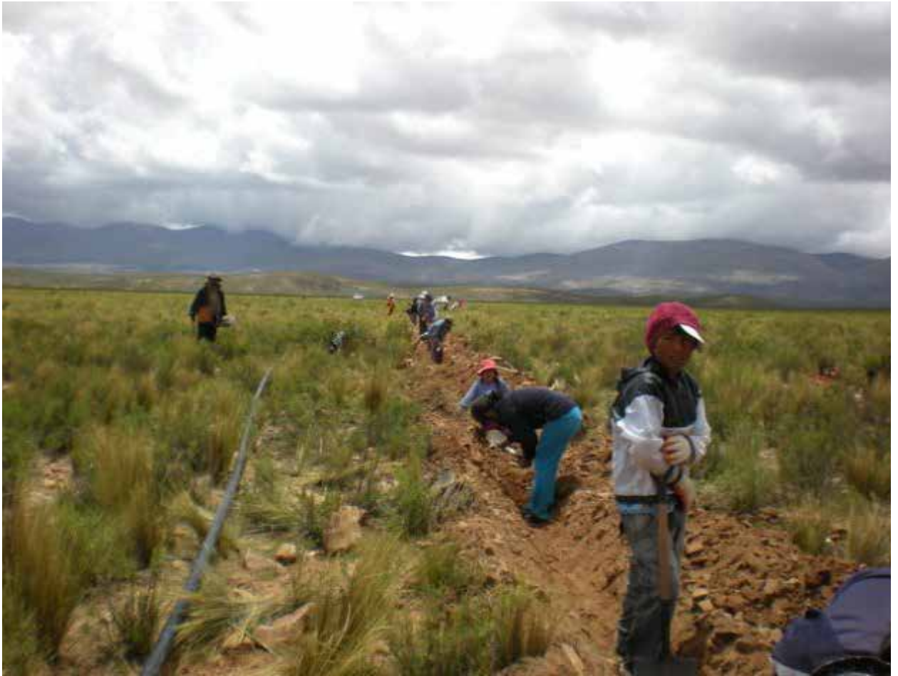
Long months of community work to install pipes to bring water from rock glaciers to indigenous villages in the Puna region in northwest Argentina served to strengthen collective organisation and community ties in an inhospitable ecoregion, where solidarity and joint efforts are essential to daily survival. Credit: Courtesy of Julio Sardina
