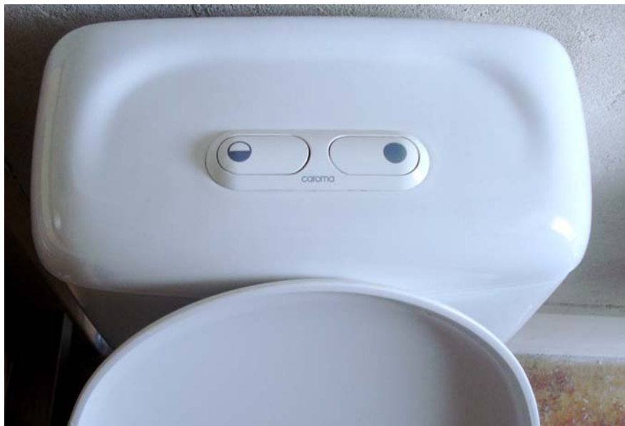
A dual flush toilet at the Ecology Action Centre's greenly renovated office in Halifax saves between 37 and 99 litres of water per day. Photo by Sadie Beaton.
